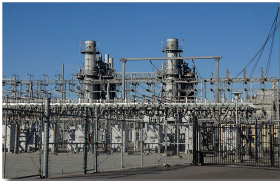
Figure 3. Modern electric infrastructure.
